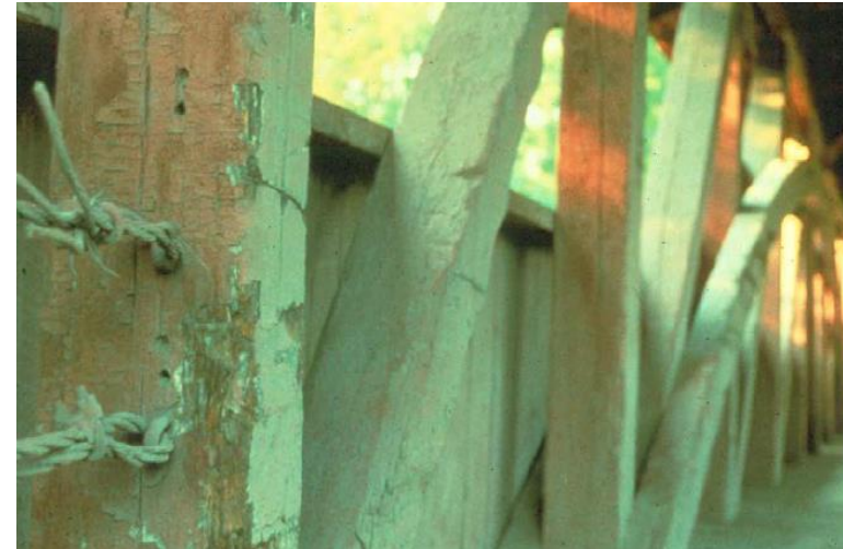
Fonte: BRIDGE INSPECTION MANUAL – NY'S DOT
