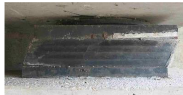
Fonte: BRIDGE INSPECTION MANUAL – NY'S DOT
