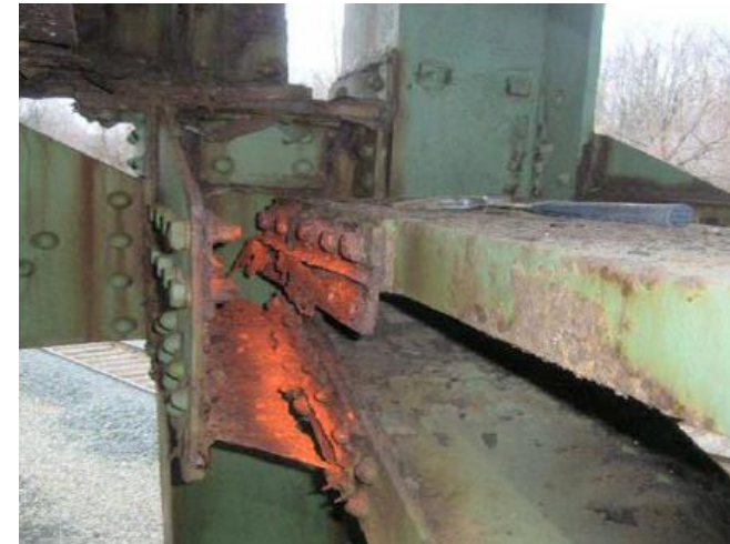
Fonte: BRIDGE INSPECTION MANUAL – NY'S DOT
