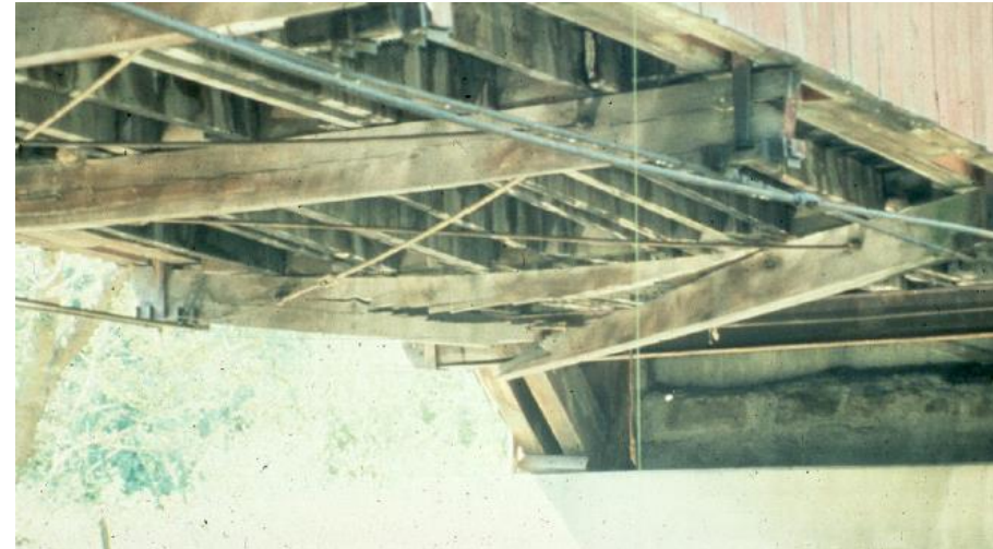
Fonte: BRIDGE INSPECTION MANUAL – NY'S DOT
