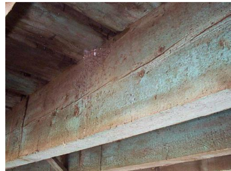
Fonte: BRIDGE INSPECTION MANUAL – NY'S DOT
