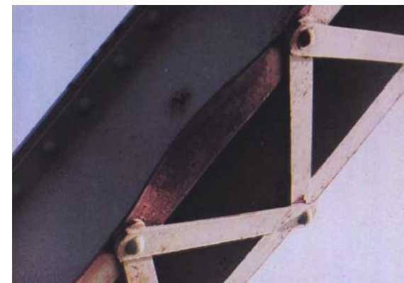
Fonte: BRIDGE INSPECTION MANUAL – NY'S DOT
